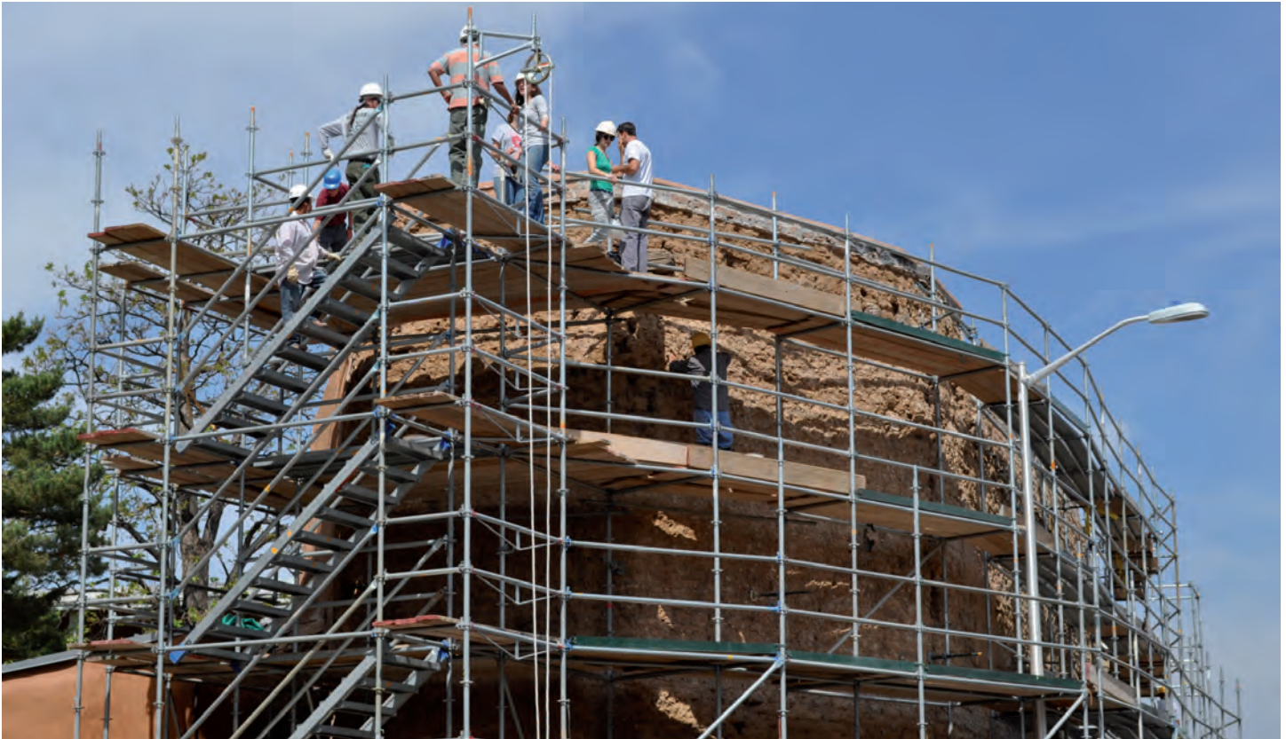
■ Connecting youth with their community. This field school focused on connecting tribal youth with their community's heritage. Here the trainees are participating in the multi-year rehabilitation of San Miguel Chapel, Santa Fe, New Mexico. ( Jake Barrow/Cornerstones Community Partnerships )
