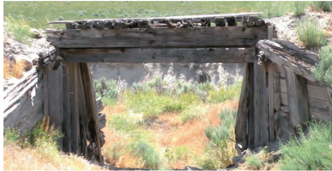
Left, the University of Vermont team restored a trestle at Golden Spike National Historic Site, shown before, during, and after restoration. (Randall Skeirik/National Park Service Vanishing Treasures Program)
